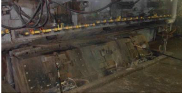
Figure 1. Old style large hood covering three spouts
