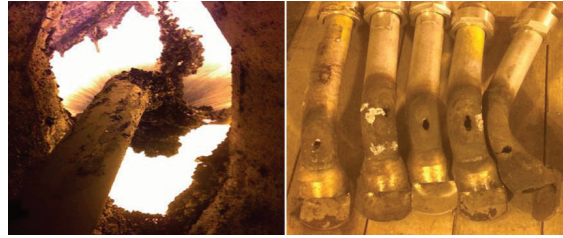
Figure 8. Liquor and ash accumulation on liquor nozzle (left), damaged nozzles from overheating (right)
