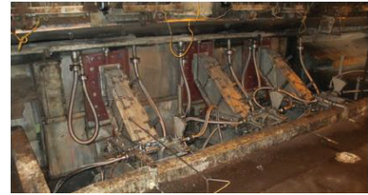
Figure 4. Large hood replaced by 3 individual spout hoods
