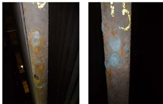
Figure 13. Corroded tertiary superheater tubes.
